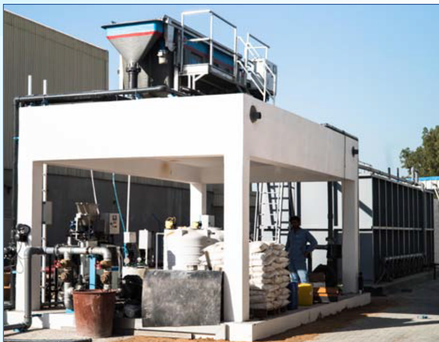
EfloDAF in operation as pre-treatment to an EfloSAF. Typical industrial waste water application for a textiles factory producing a mixed waste water including dyes and organic matter.
